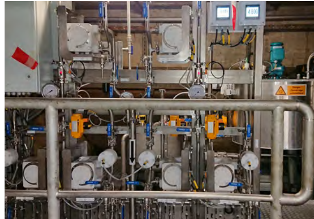
QUANTUM pumps for acid mix transfer (Belgium)
