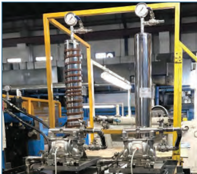
ASTRAevo FOOD pumps (1/2" metallic version) installed at PHARMASYSTEMS (Europe).
