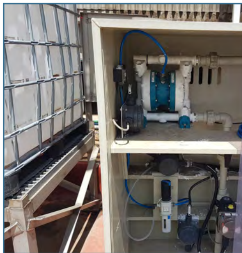
ASTRAevo pumps (1/2" PP+glass version) installed for chemical transfer (Europe).
